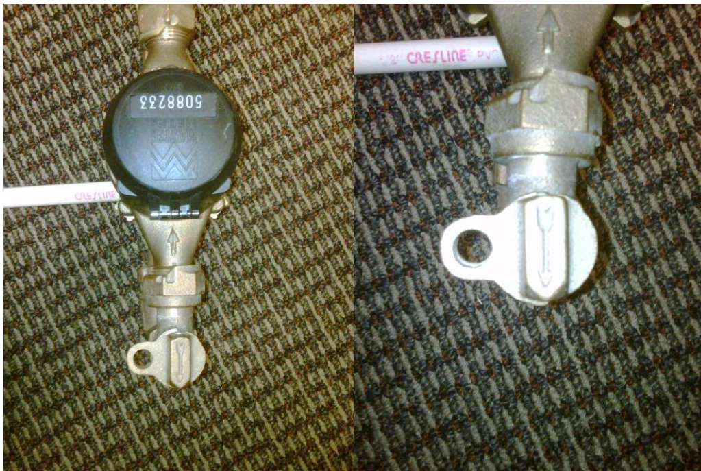
The pictures above show the cut-off valve in the off position.
